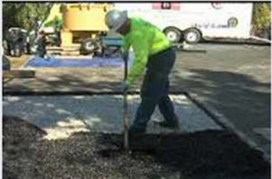
A city worker lays Flexi-Pave in a parking lot in downtown Dunedin.
